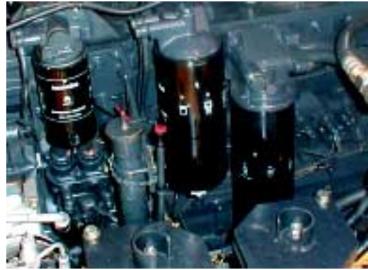
Photo 12 Centralized filter elements
